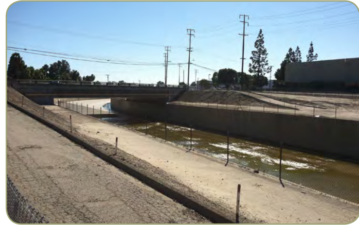
Figure 3.8: Looking south towards the Artesia Boulevard Overpass, Service Roads, and Coyote Creek Box Channel
