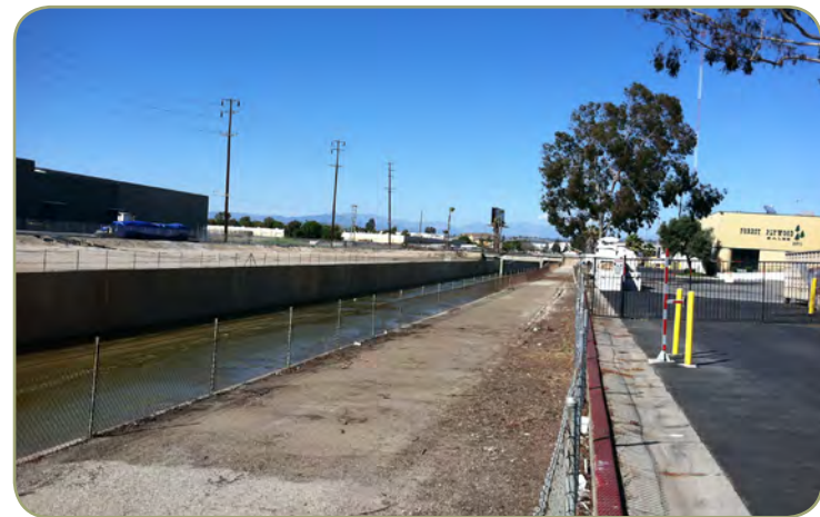
Figure 3.9: Looking north towards the UPRR Branch Line Overpass from a driveway off of Artesia Boulevard
