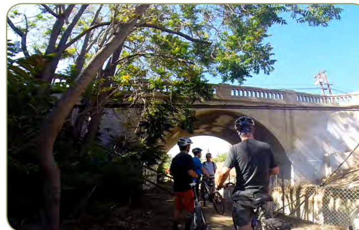
Figure 6.6: The existing Golden Avenue bridge over the channel ROW, planned for improvement.
