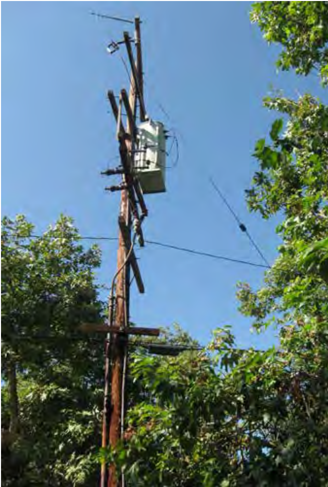
OC Zoo Overhead Electrical Utility
