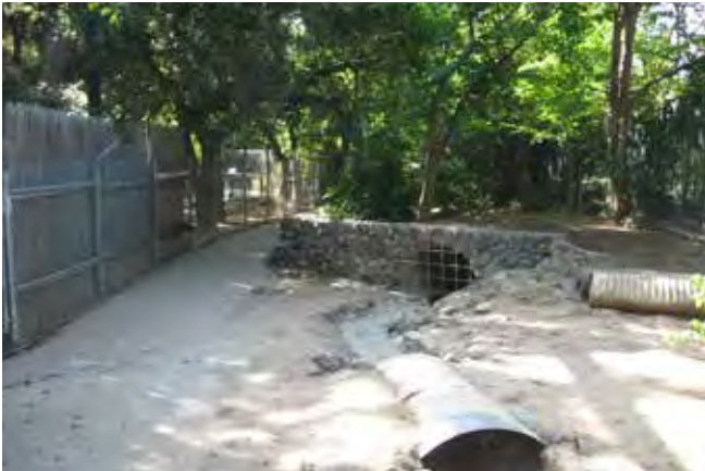
OC Zoo Drainage Facility
