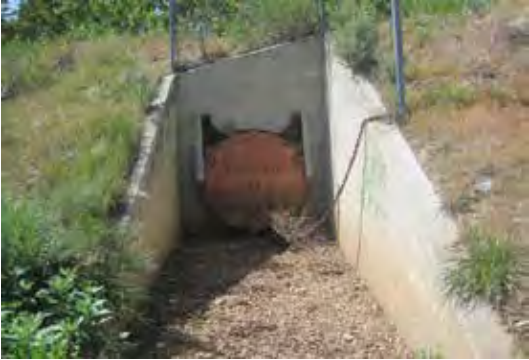
C Flap gate Drainage Outlet at Santiago Creek
